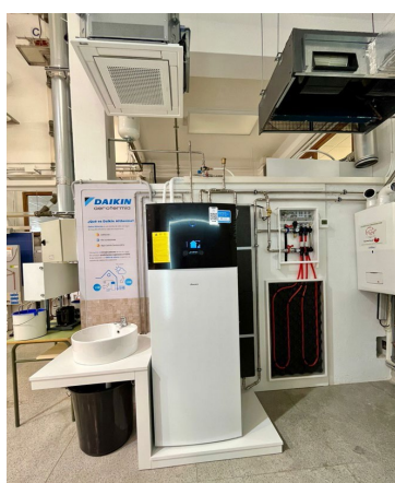
Imagen. Showroom Aerotermia DAIKIN.
